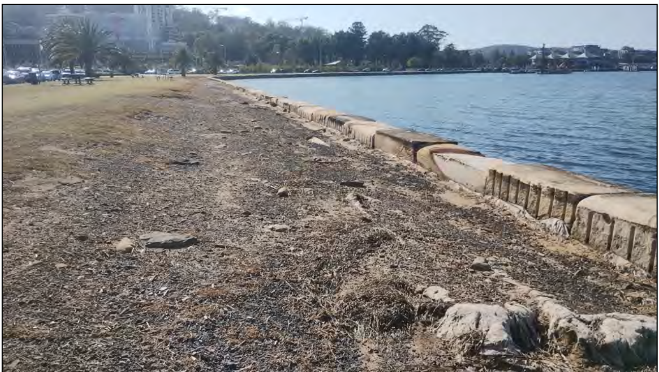
Photo P1-8: Exposed ground surface adjacent the seawall along Graham Park.
