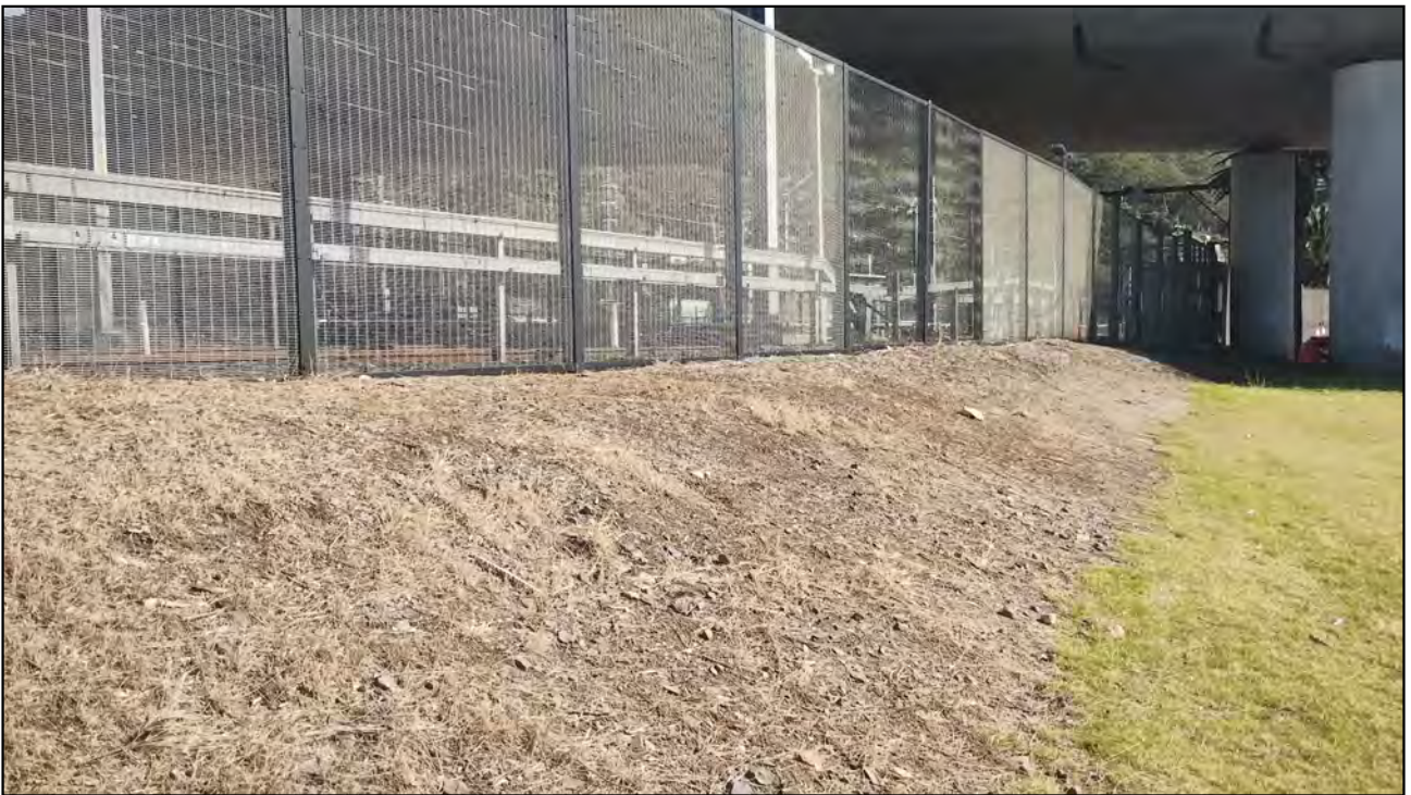
Photo P1-12: Close-up of filled mound along rail corridor.
